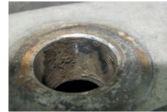
Corrosion wheel nut area
