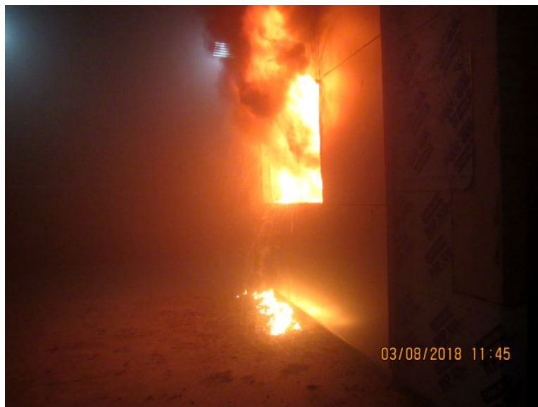
Photo No. 36 Side View of Panel Consumption
