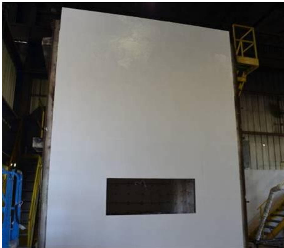
Figure B-2. Wall Assembly following Application of DuPont™ Tyvek® Fluid Applied WB.
