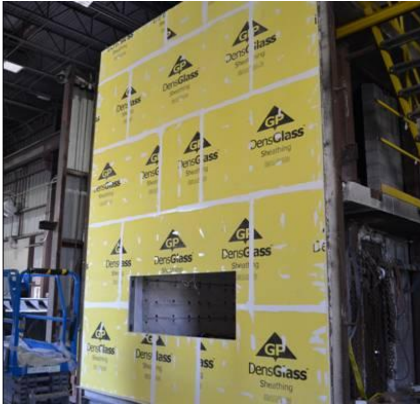
Figure B-1. Base Wall with Application of DuPont™ Tyvek® Fluid Applied Flashing and Joint Compound over Sheathing Joints and Fastener Heads.
